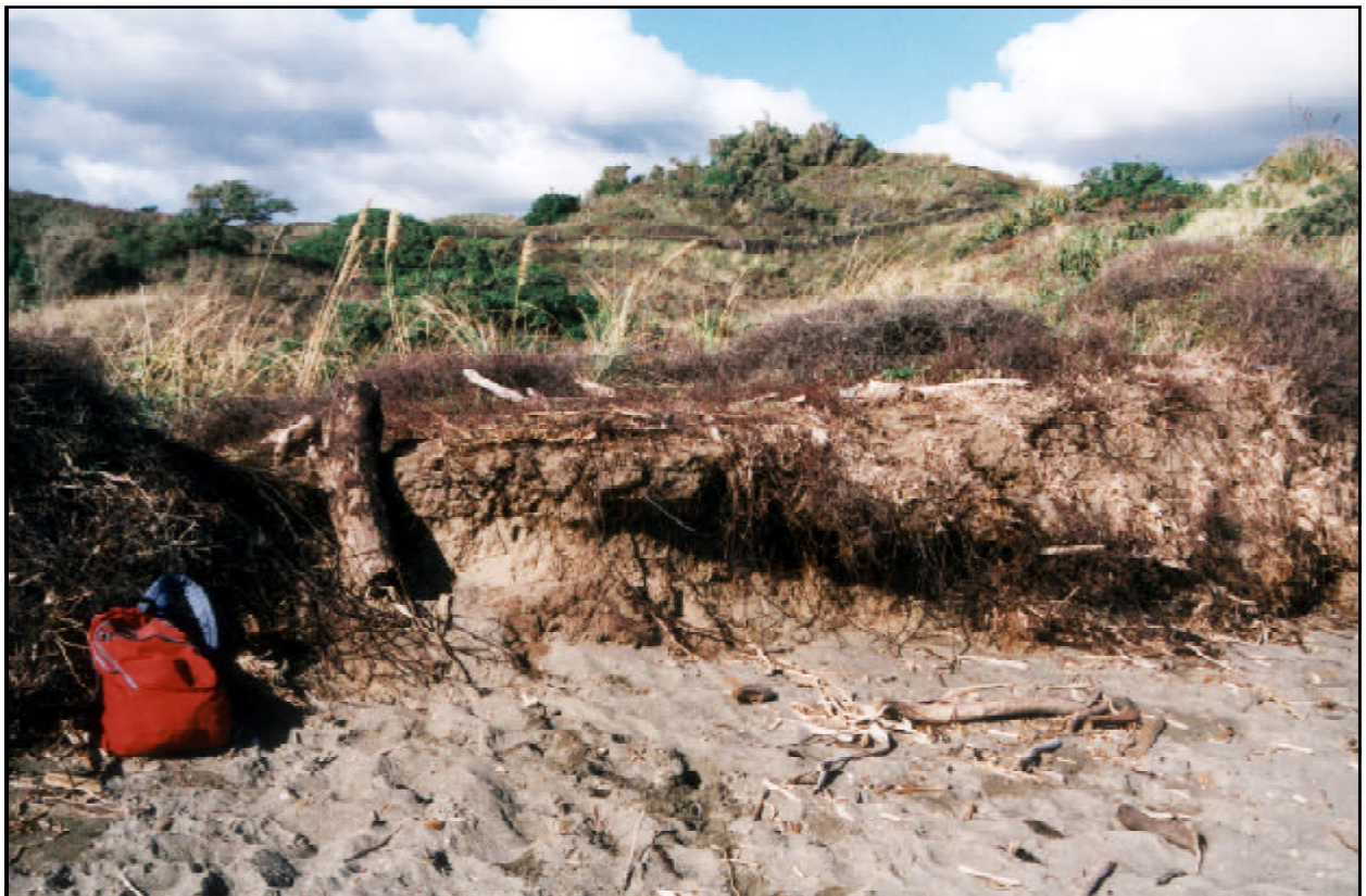
PHOTOGRAPH 10: Simple wooden stepped access could be provided here to avoid erosion at nick-point (behind log) which is present step down point.
