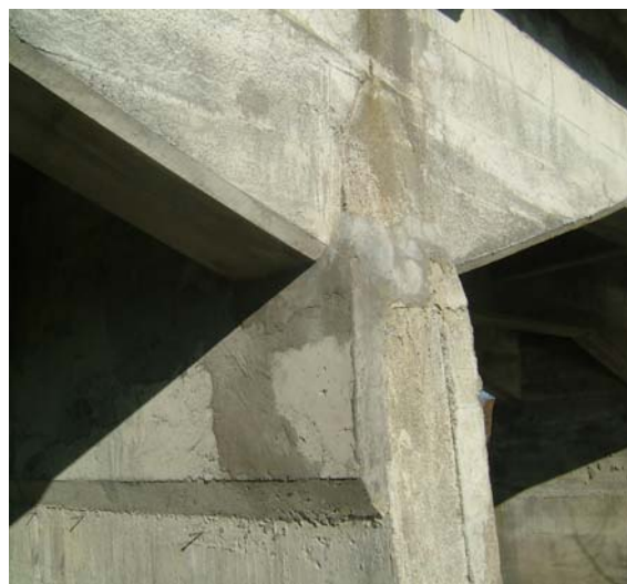
Figure 3. Repairs to the crack at the hinge point at the top of the piers are still obvious.
