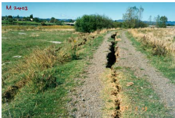
Figure 6. Liquefaction damage to stopbank Whakatane River, left bank. The Landing Bridge is in the background and Whakatane is to the left of the photograph. Note the evidence of sand boils on the river berm to the left.
