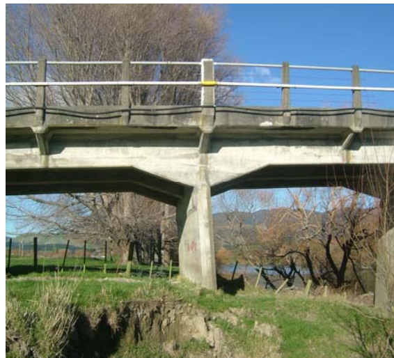
Figure 2. Out of plumb pier to the approach spans of the Lower Valley Bridge (Tuhitarata) due to lateral spreading during the 1942 Wairarapa earthquakes of June or August. (Most likely June)
