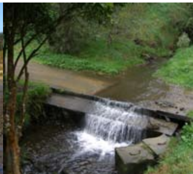
Stream crossing of Mitchell Stream at Park constitutes a significant fish barrier
