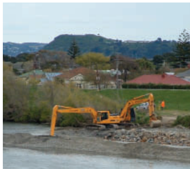
Construction of a rockline to form a new river channel edge on the Hutt River opposite Strand Park in 2004. The gravel bund in the river helps reduce sediment input into the river during construction.
