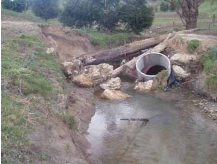
Illegal works in the Kopuaranga Stream
