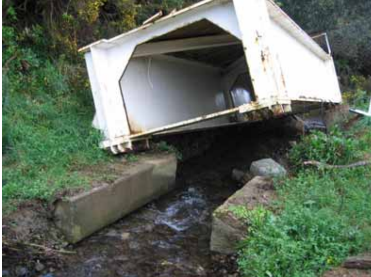
Unauthorised culvert and associated structures in Mitchell Stream, Porirua
