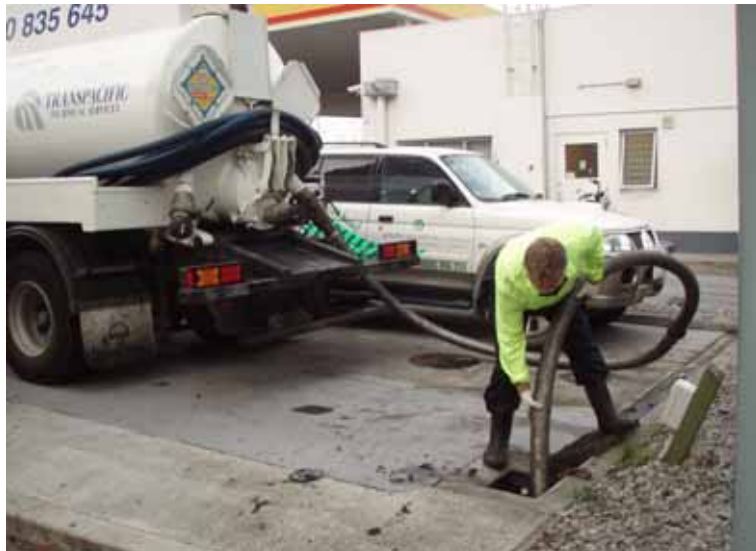
A stormwater sump being cleaned out after a hydrocarbon spill at Shell Thorndon
