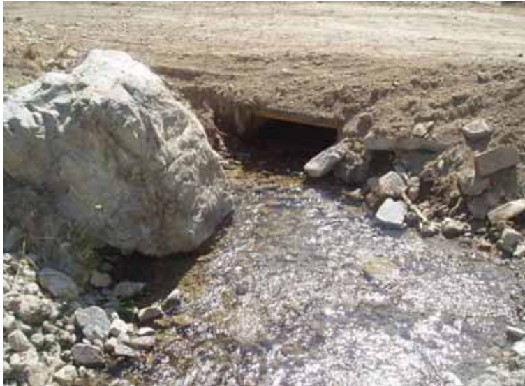
An illegal culvert on Moonshine Hill Road
