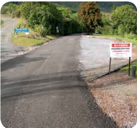
Millings were laid on the Tunnel Gully entrance road to create a hard surface
