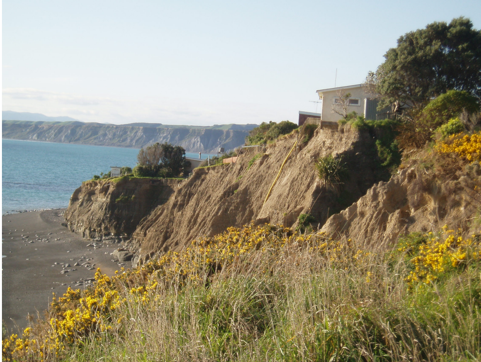
Figure 7: Photograph showing the high erosion risk of a subdivision in Whatarangi, Wairarapa 18
