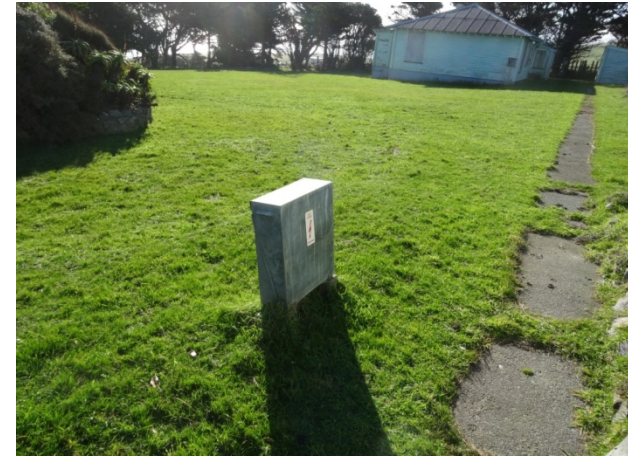
Fuse box in front of Power House
