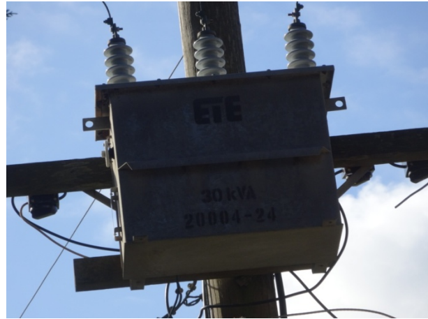
30kVA pole mounted transformer
