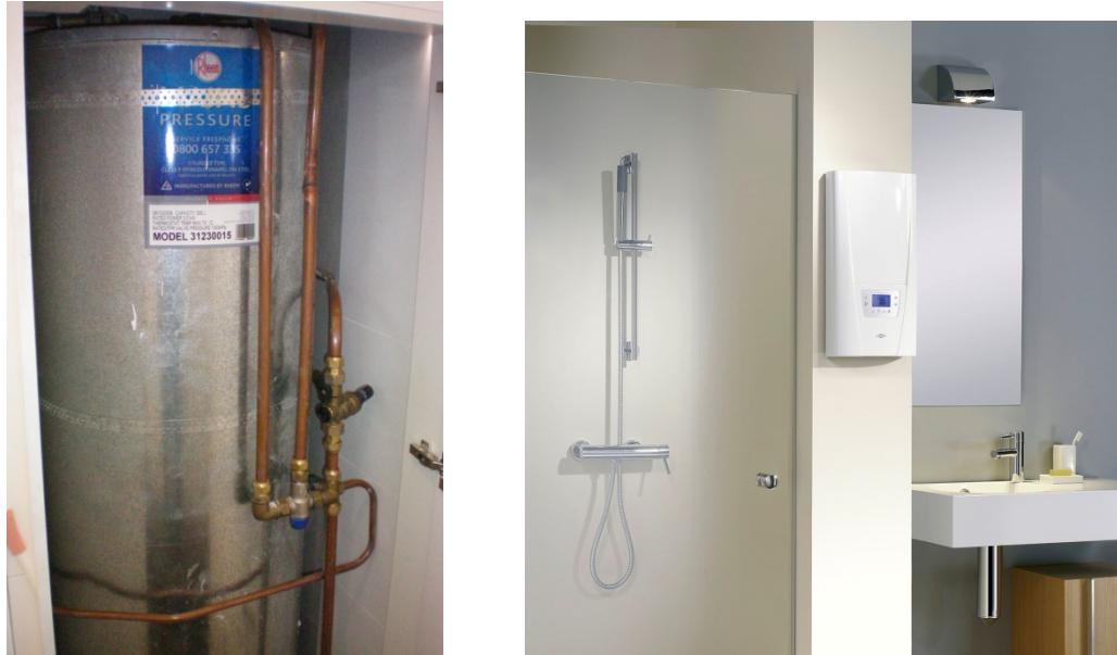
Figure 2 – Electric Hot Water Cylinder and an Instantaneous Electric Hot Water Heater
