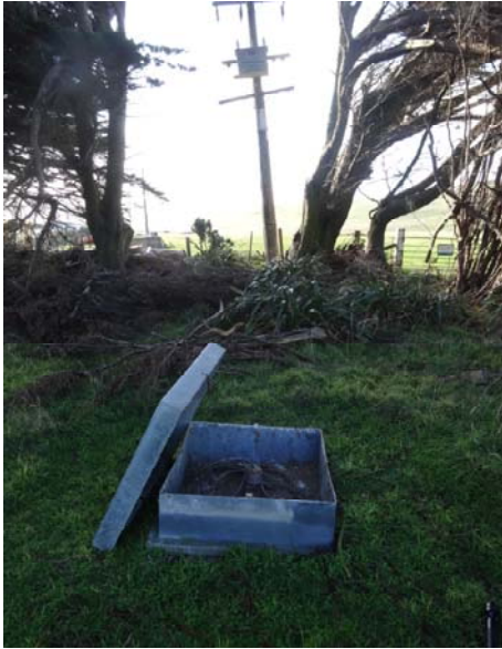
Pole with transformer in background. In ground cable manhole in front
