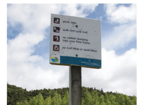
Top: Existing warning signage relating to toxic algae has become damaged due to wind and weather
