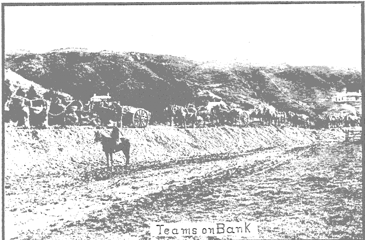
Plate 27: Construction of the first stopbanks - compaction. Source: Alexander Turnbull Library, York Studios, neg. F28346
