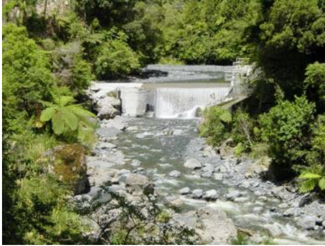
Orongorongo Weir and water intake, Orongorongo River. Assets such as weirs are being progressively seismically strengthened via asset renewal programmes.
