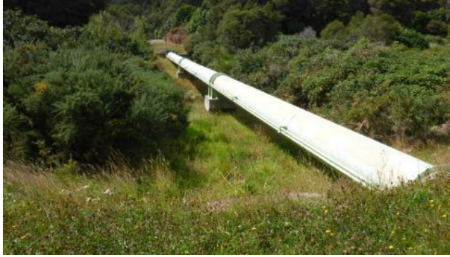
Raw water supply pipeline upstream of the Wainuiomata Water Treatment Plant
