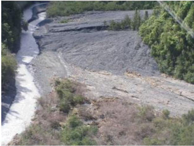
River bank and asset protection measures such as gabion rock baskets are utilised as flood and erosion stabilisation measures
