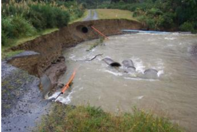
A storm in the Wainuiomata catchment downstream of the intake in 2005 caused heavy erosion of an access road and broke water supply pipe and power cable.
