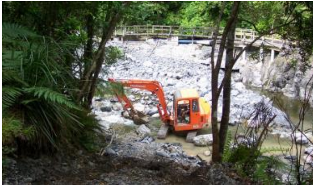
Orongorongo River track and pipeline repair works in 2005. With severe rain events expected to become more frequent, works to strengthen and reinforce assets such as access tracks and water pipelines are required.
