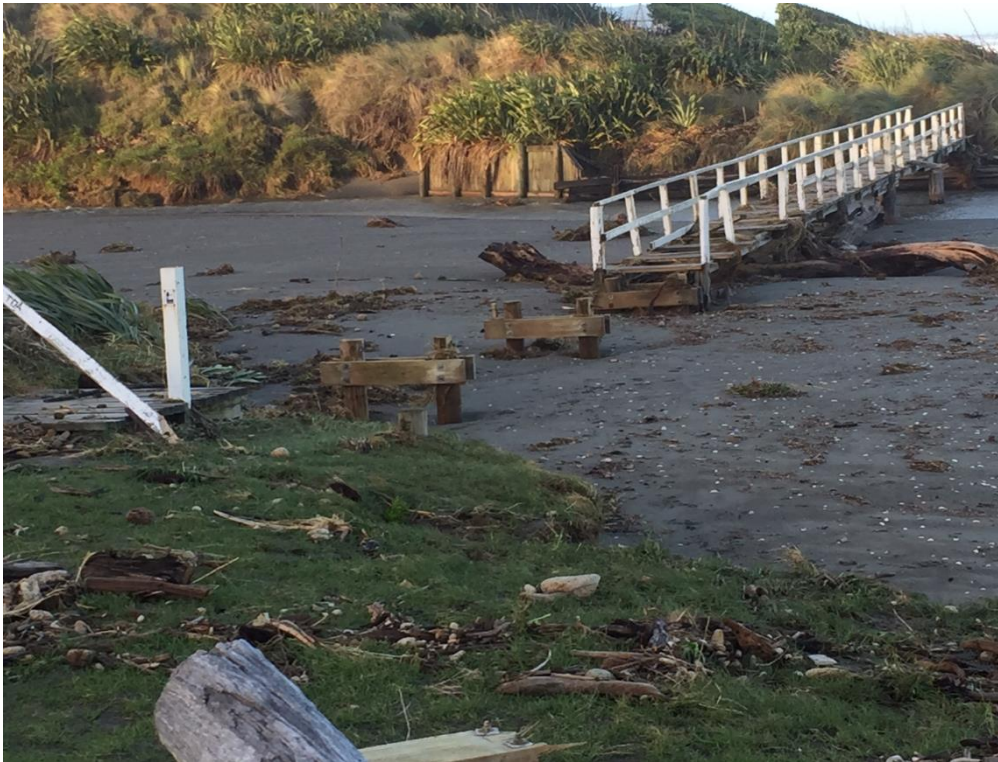
Storm damage after ex Cyclone Gita at the Wainui Stream mouth, Queen Elizabeth Park in February 2018. For safety reasons the remaining sections of the bridge were removed.
