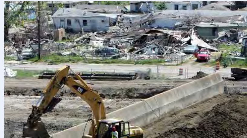
Flood recovery from another breached levy – Hurricane Katrina
