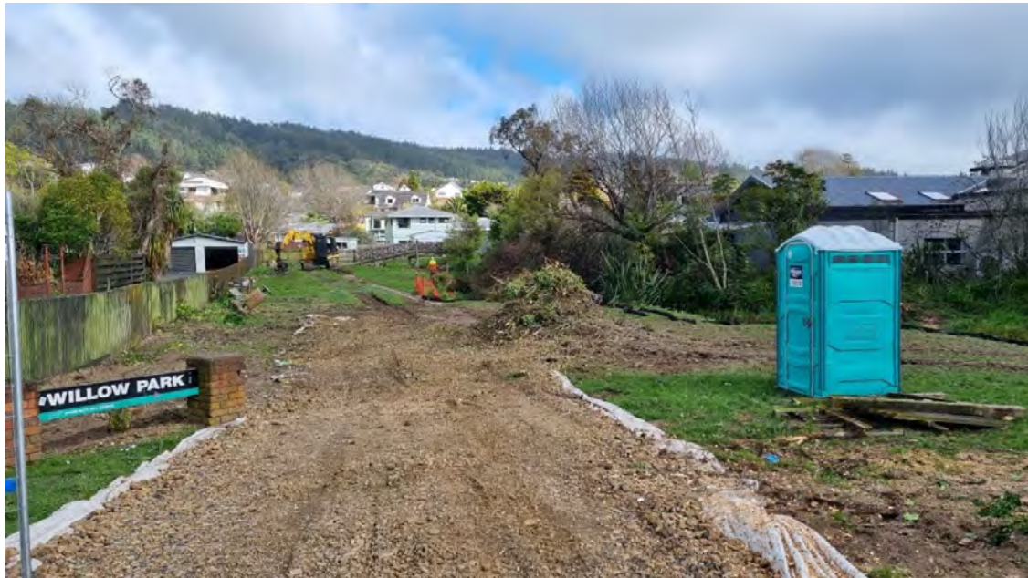
Figure 2: Willow Park vegetation clearance and setup for stream bank upgrades (photo credit: GHD)
