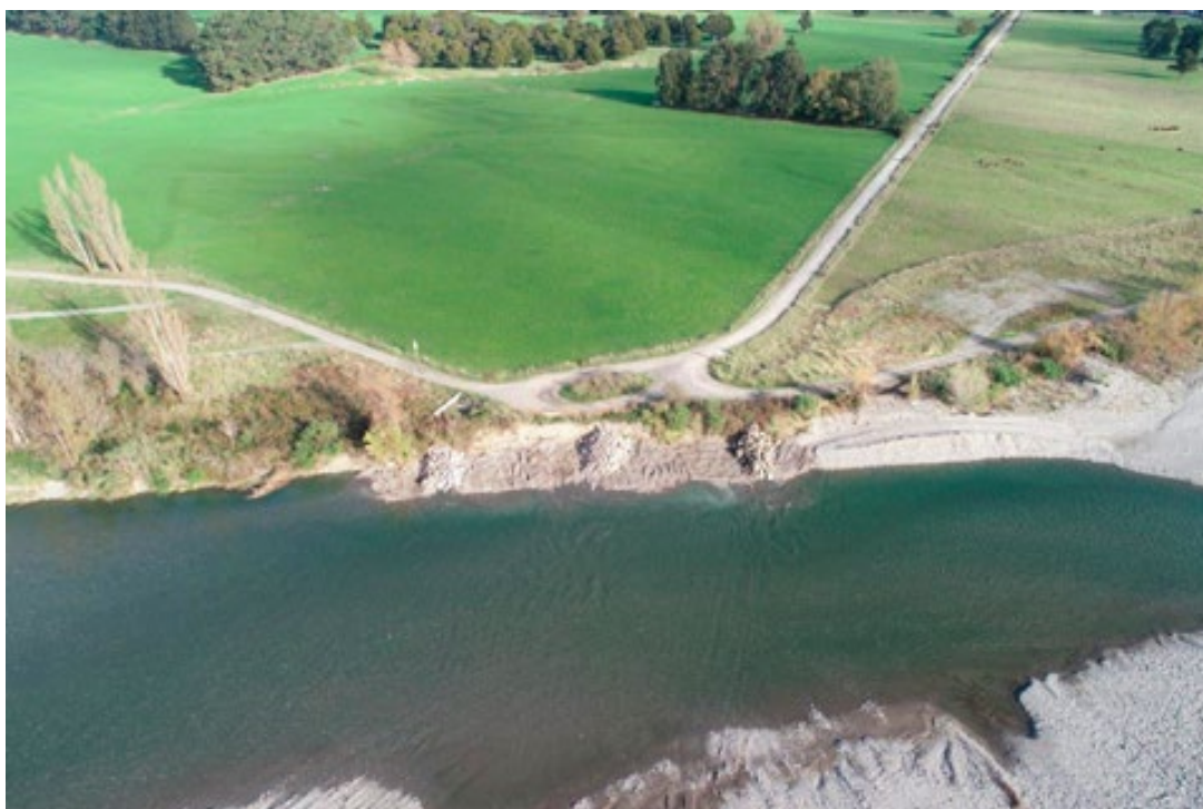
Figure 88: Critical Area Photograph – Kuratawhiti Street – GWRC.
