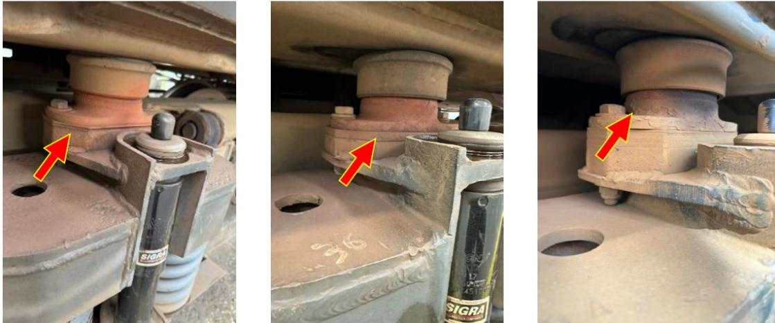
Red-coloured side bearers being found across the fleet. The red is indicative of iron fretting
