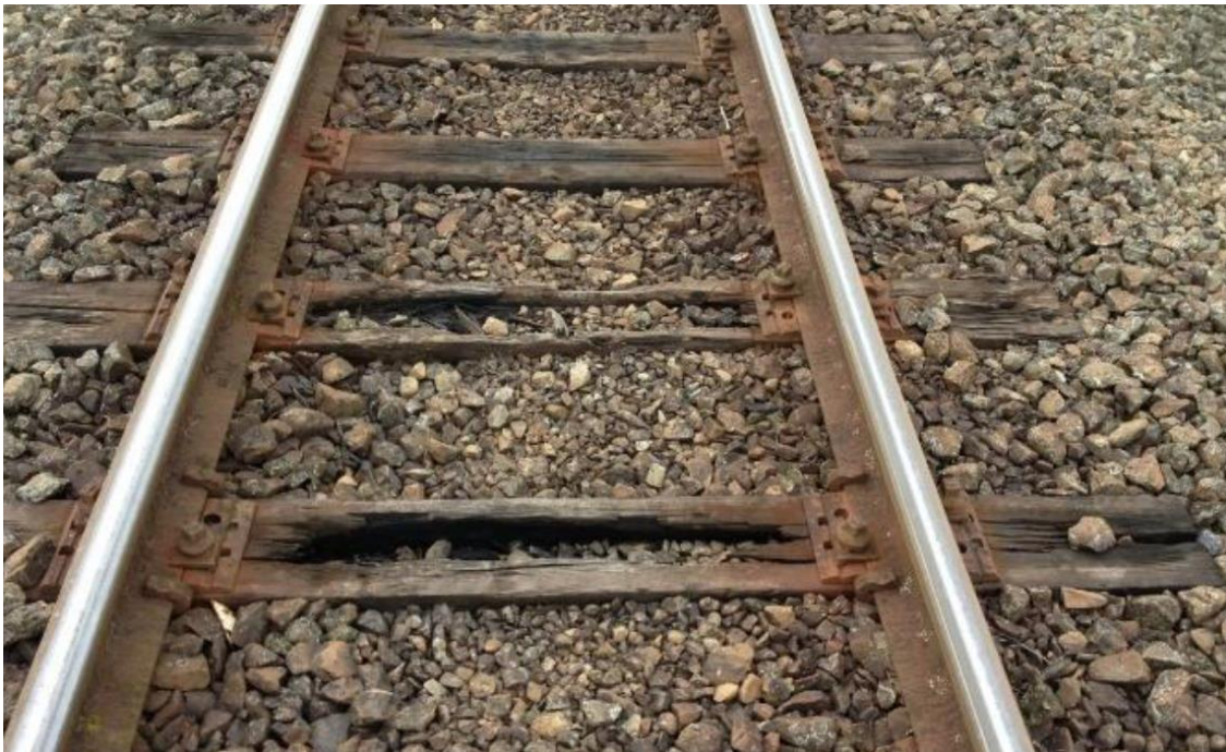
Figure 1. From Single Stage Business Case, “deteriorated Treated Pinus Radiata (TPR) sleepers. These are endemic on the Wairarapa Line, with the sleepers replaced during significant volumes of renewals nearly 40 years ago now having run through their life cycle”
