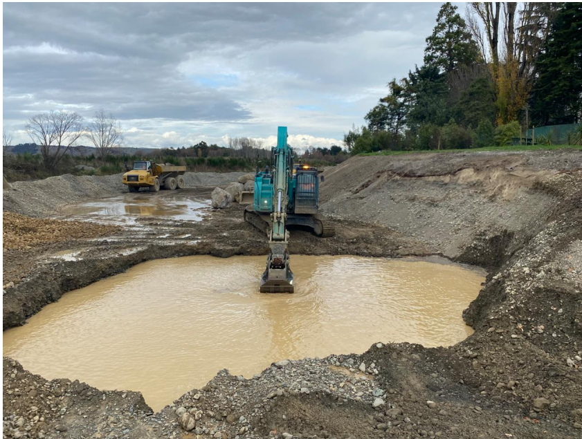
Figure 6: Stage two (Waipoua River) – Excavation of the rock revetment within the Waipoua River (the excavation is banded from the Waipoua River and is not within the flow of the river)
