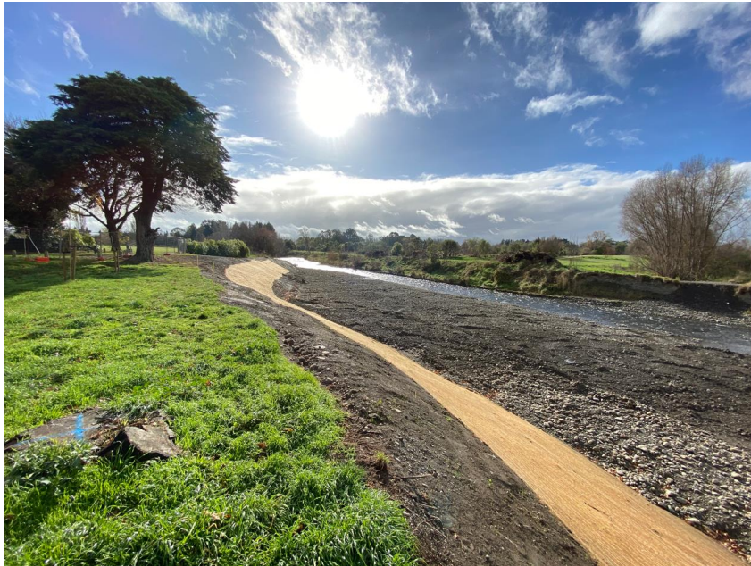
Figure 7: Stage two (Waipoua River) – Rock groyne and rock revetment completion within the Waipoua River. Coconut matting has been installed to the battered river bank above the rock revetment
