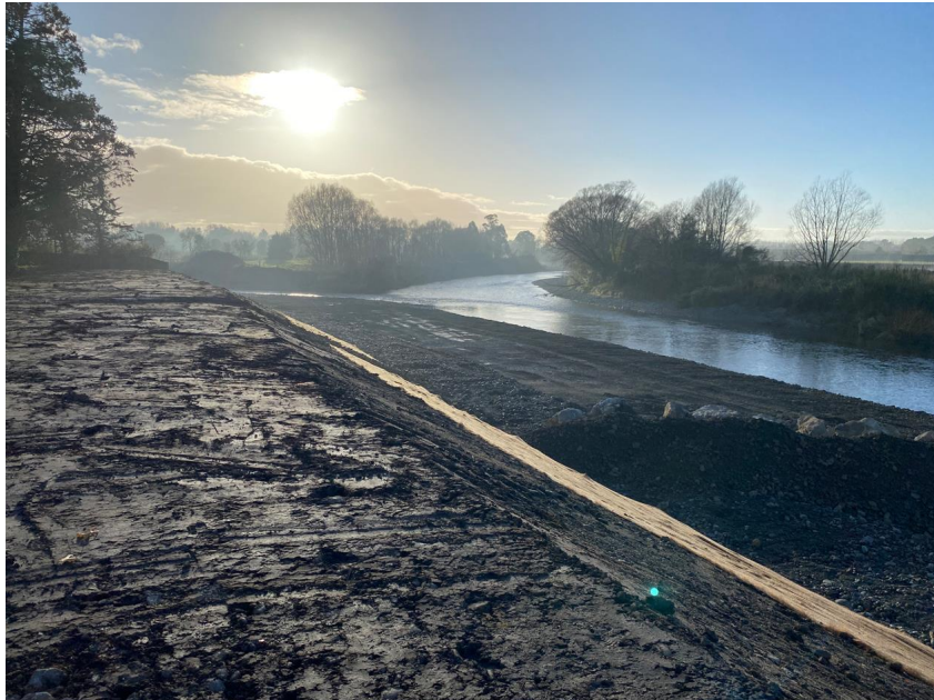
Figure 11: Stage two (Ruamāhanga River) – A section of the rock revetment within the Ruamāhanga River is completed. The temporary bunding has been retreated. This photo overlooks the confluence of the Waipoua and Ruamāhanga Rivers
