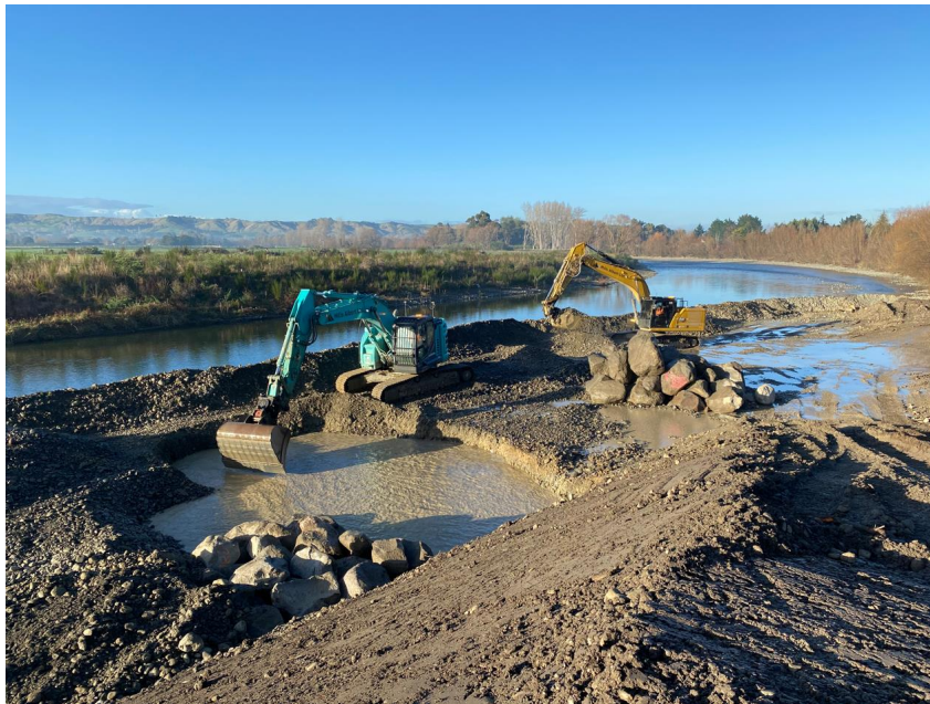
Figure 10: Stage two (Ruamāhanga River) – Excavation of the rock revetment within the Ruamāhanga River (the excavation is bunded from the Ruamāhanga River and is not within the flow of the river)
