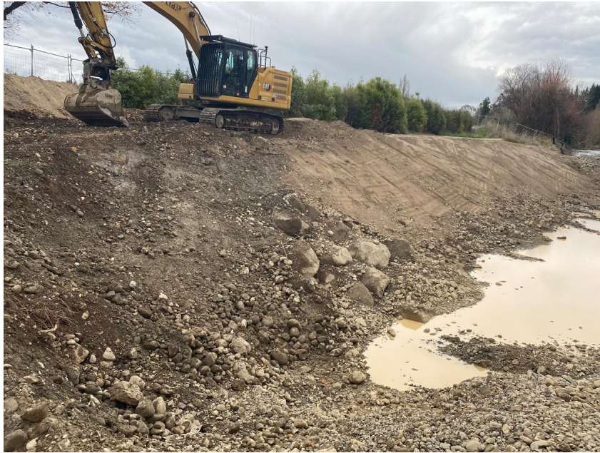
Figure 5: Stage two (Waipoua River) – 1,000 tonne rock groyne completed within the Waipoua River
